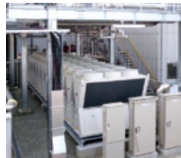
▲ Equipment to treat and reuse the water used in industrial processes.
