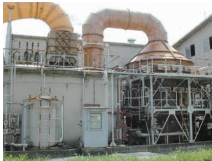
Gas emission washing treatment facility (Tokushima Plant (Kitajima location))
